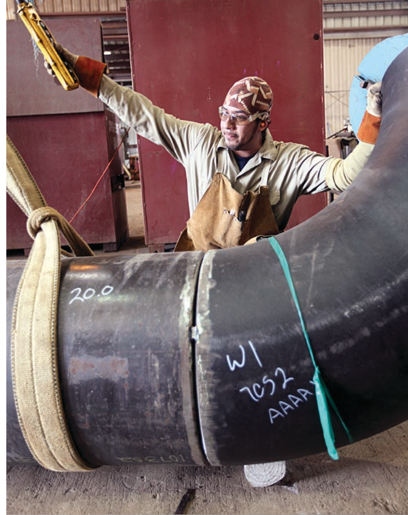
Pipe Welder Jaime Coronado rigs a pipe into position for welding in one of the Freeport fabrication shops. Photos/Alissa Rosebrough
