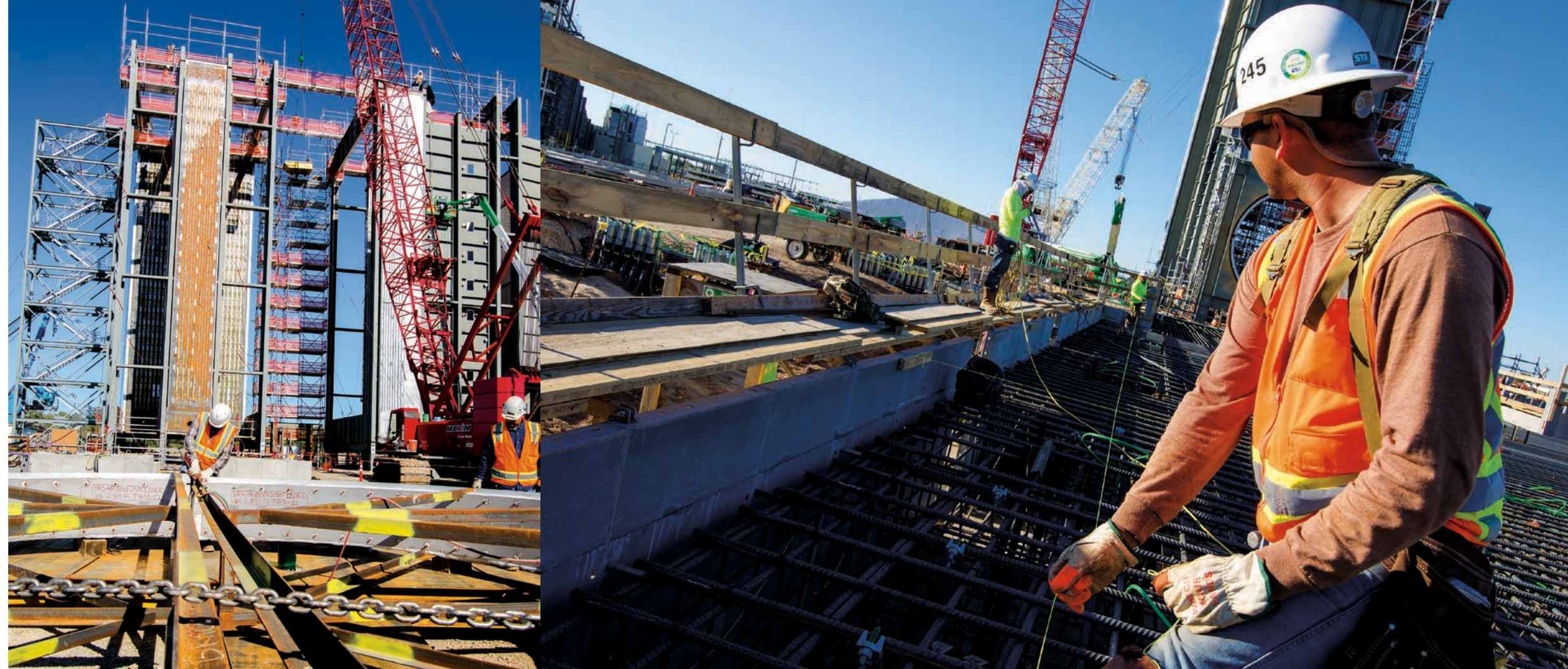
Above: In November and December, the projects began putting up pipe racks and preparing to receive steam turbine generator sets in the first quarter of 2016.
