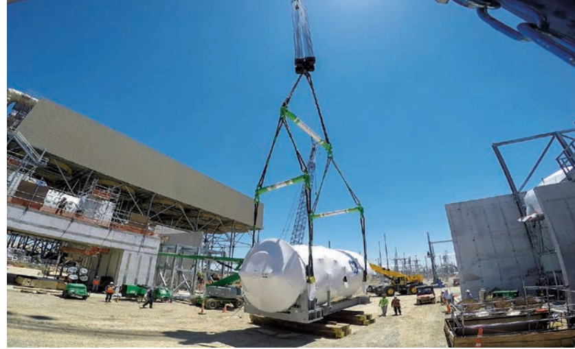
The turbine blades within this precious package will soon be spinning, turning natural gas into megawatts at the Wolf Hollow Project in Granbury, Texas. Photo/Zachary Spence
