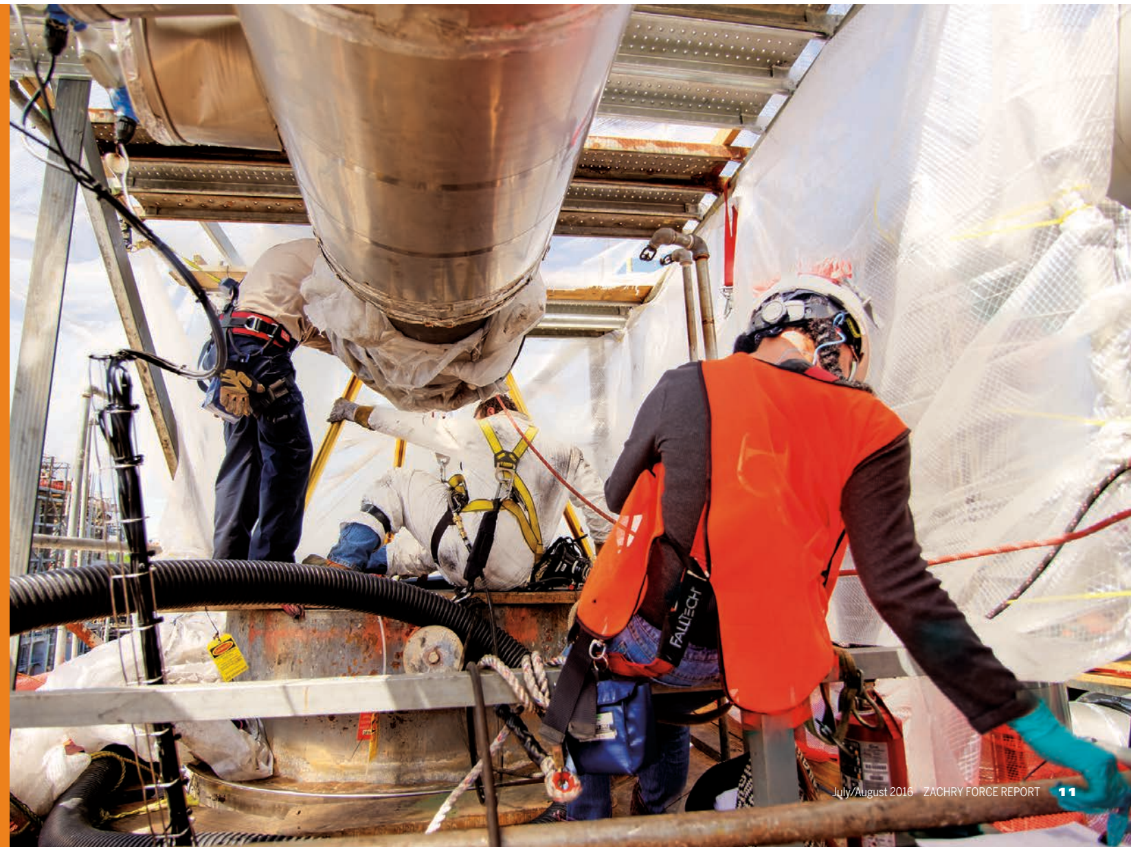
Zachry's Tyler Anderson Thomas emerges from a catalyst reactor tank after completing welding work inside. The team was prepping the tank for catalyst loading later that evening. Seated in the foreground is JVIC Firewatcher Brandi Boudreaux.
