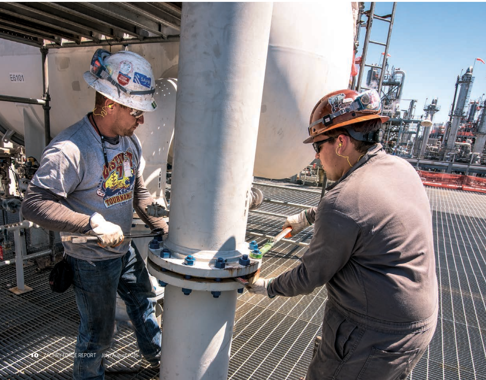
JVIC Boilermakers Jacob Hughes and George Kilsby change out bolts on a flange at the BASF plant in Geismar, Louisiana. Photos/Nick Grancharoff
