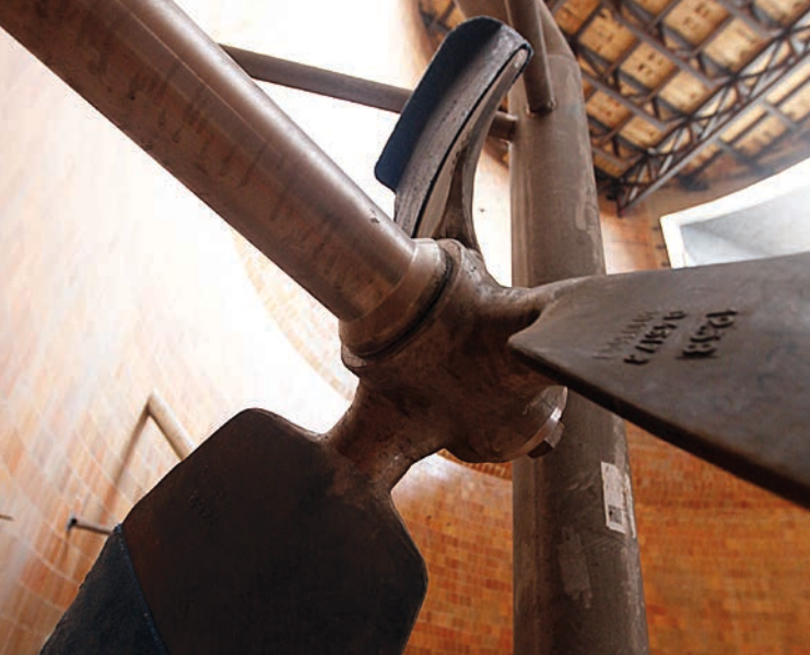
An absorber module agitator blade viewed from inside an absorber, or scrubber, that is one of three scrubbers being erected at the plant. Photos/Alissa Hollimon
