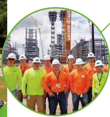
A group of Zachry's engineering interns visited the CPChem polyethylene plant project site in Brazoria County, Texas, over the summer. Photo/Russell Epperly
