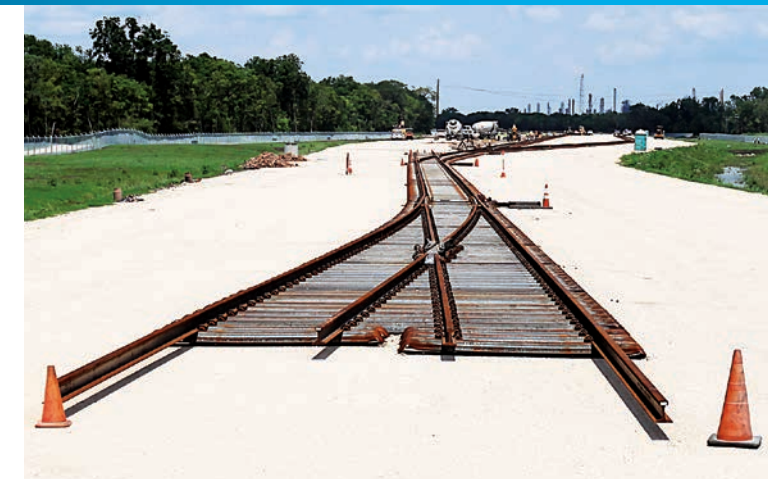
The polyethylene plant will be linked to a Union Pacific Class 1 rail main line, allowing product to be picked up inside the plant and transported in either an eastbound or westbound direction.
